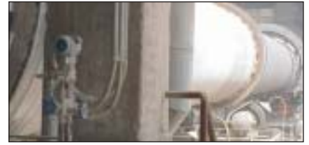
Figure 9: 100 of the 238 transmitters on the new kiln line are intelligent ones with HART digital communication capability, such as this Rosemount® Model 3051 differential pressure transmitter
