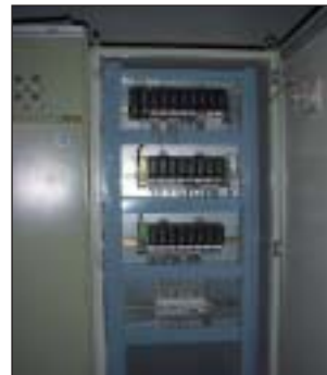
Figure 5: DeltaV controller assembly for the cement mill dust collector, seen at far right in the network diagram (see Figure 6 for identification of modules)
