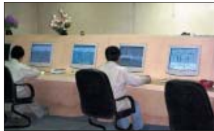
Figure 7: DeltaV operator and engineering stations in the control room
