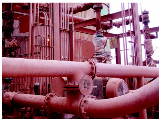
CVG Bauxilum plant entrance with Rosemount High Signal Flowmeter system installed
